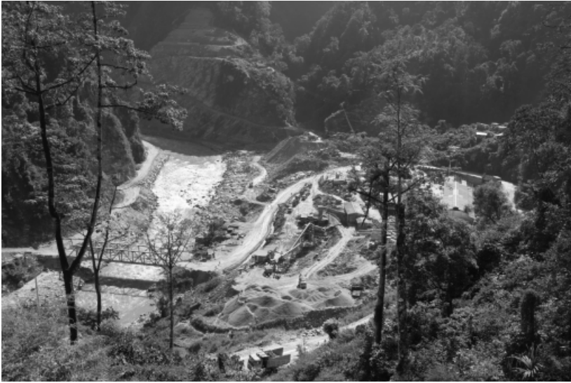
Figure 3.2. The construction site of the Arun-3 hydropower project in Nepal, November 2019. © Matthäus Rest.
